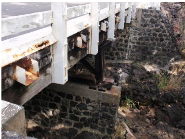
Hilea Bridge along Mamalahoa Highway is over 50 years old and needs to be rehabilitated or replaced.
