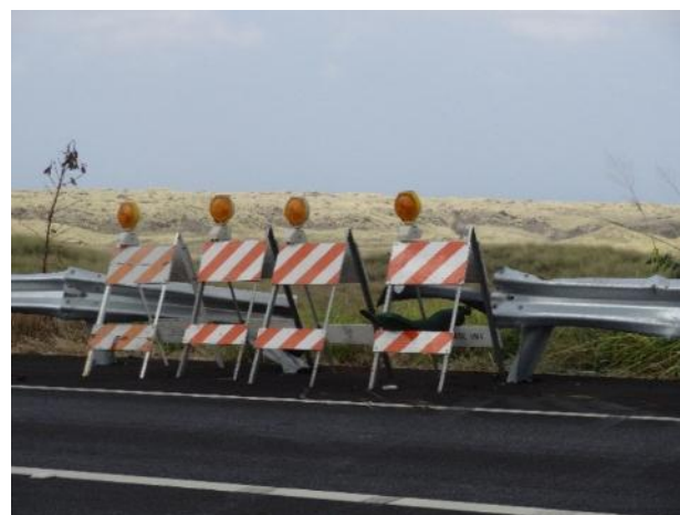
A guardrail is in need of repair.
