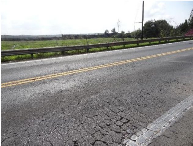
Pavement resurfacing will be required along Kawaihae Road.
